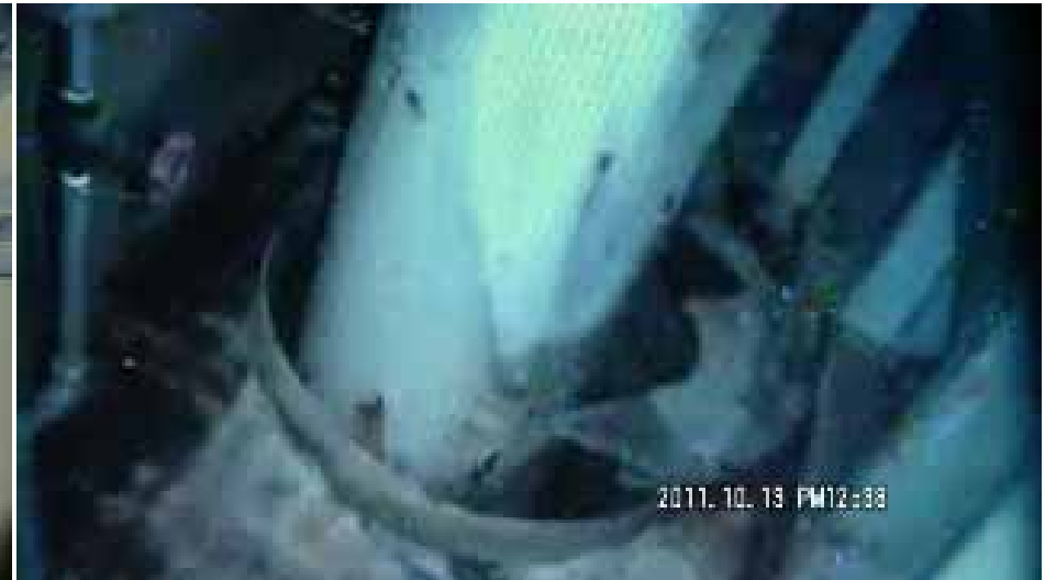
Situation of the penetration on 1 st floor with no steam release (photo as at Oct. 13)
