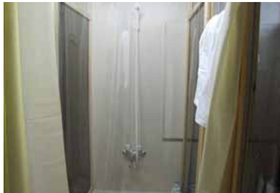
Shower room in gymnasium at Fukushima Daini
